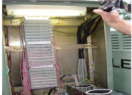
CCF cables installed behind Krone Frame supporting bars.
