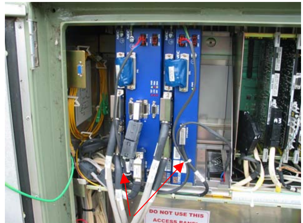
Power cables tied to BEU cable to reduce strain on power plugs
