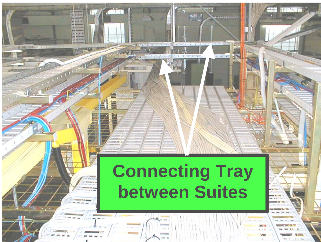
Photo 2 Signal Cable on the Teltray Planar Shelf
