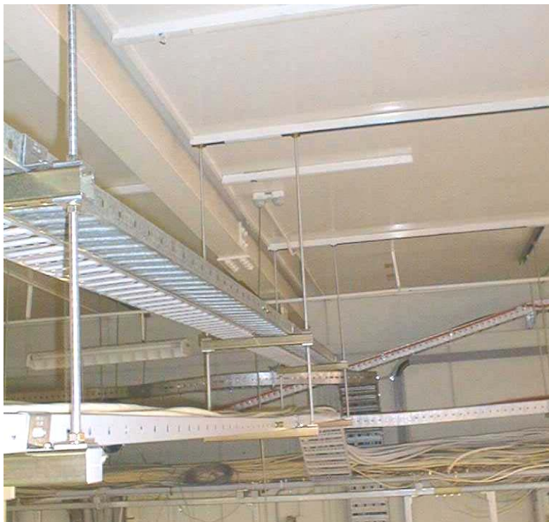
Photo 3 External TEBA Cable Runways
